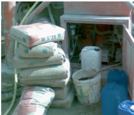
Mechanical system for metering Mapescreed 704
